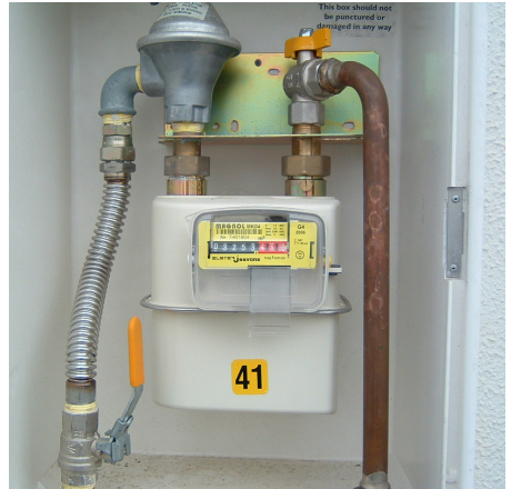
Internals of a meter box
