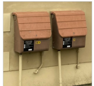
Surface mounted meter boxes
