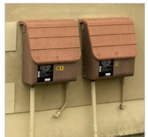
Surface mounted meter boxes
