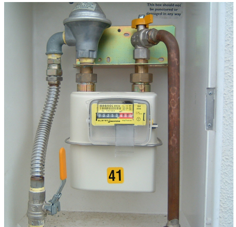
Internals of a meter box
