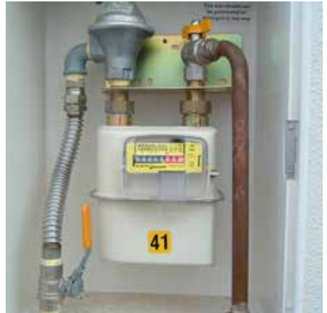
Internals of a meter box
