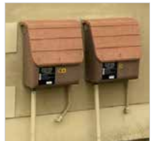
Surface mounted meter boxes
